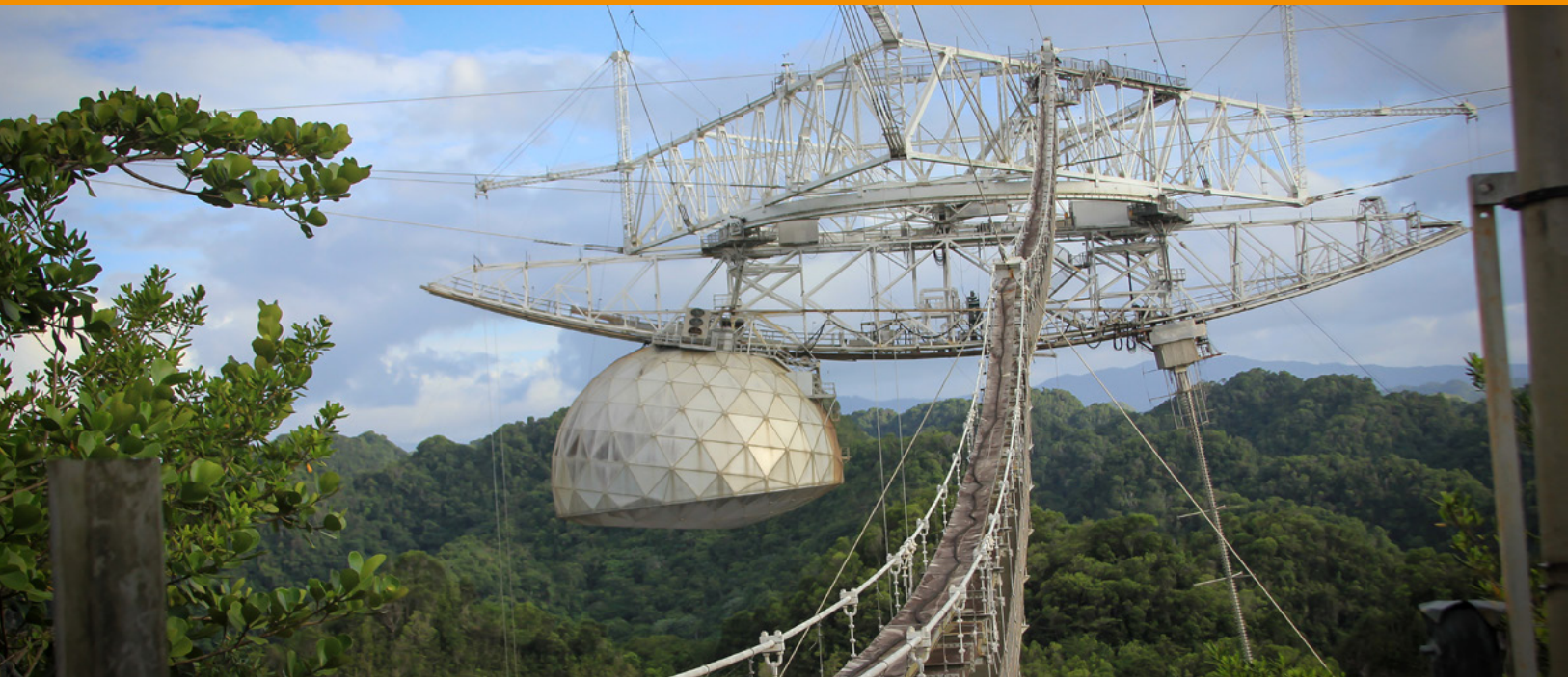
▲ The receiver platform was suspended 150m above the dish. On 1st December 2020, several cables broke and the main telescope collapsed.
